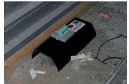
Fig 2: GT sensor mounted on upturned gutter
